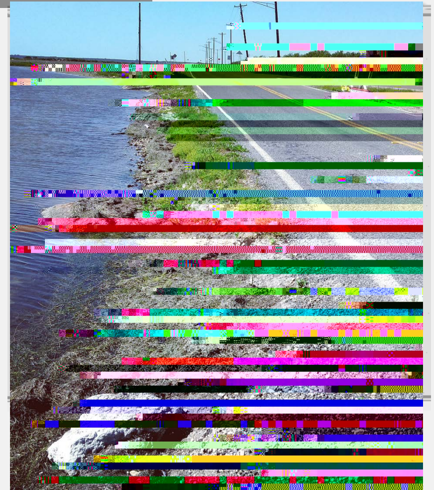
Closeup, note the irregular edge of pavement
